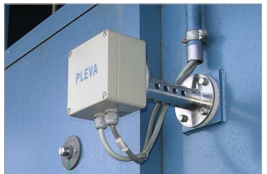
Exhaust humidity sensor FS91-S installed at the side of the relax dryer.
