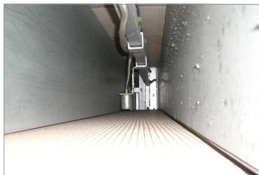
Fabric temperature sensor TDS95 installed in the dryer above the conveyor belt.
