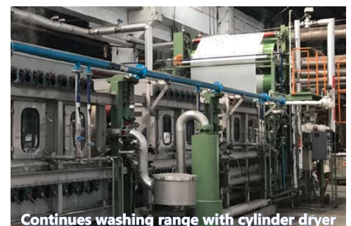
DrumDry Control at inlet of a washing range
